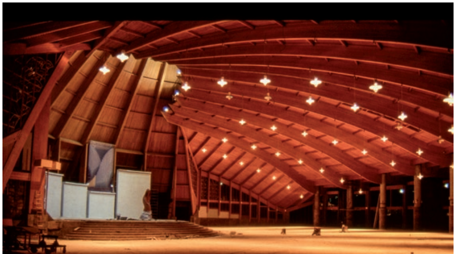
Glued laminated indoor structure at the Mary Queen of the Apostles Basilica in Yaoundé (Cameroon). Photo J. Uhalde, UBC.
