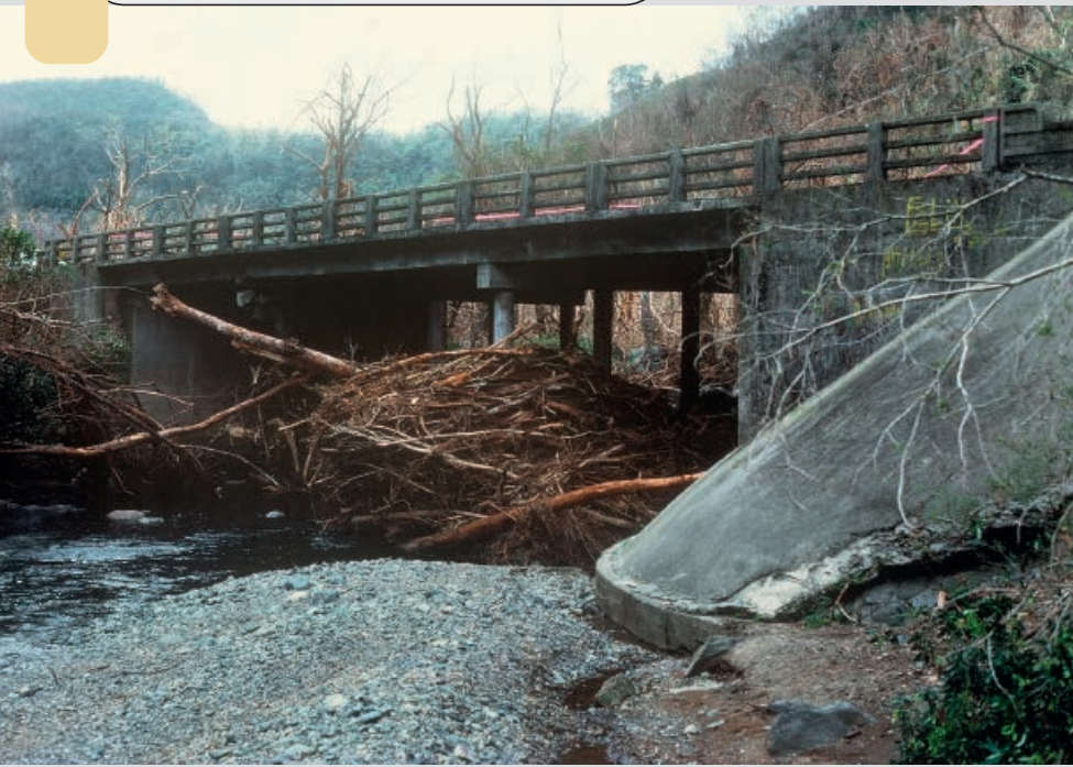
Río Mameyes: The Río Mameyes, the largest of 10 major streams that originate in the Luquillo Mountains, flows under Puente Roto (Broken Bridge) near the northern forest boundary several days after the passage of Hurricane Hugo. Stream channels throughout the mountains remained temporarily cluttered with fallen trees and soil causing changes in aquatic habitat. Puente Roto probably owes its interesting name to earlier storms when less stable wooden structures spanned the river. Photograph P. L. Weaver.
