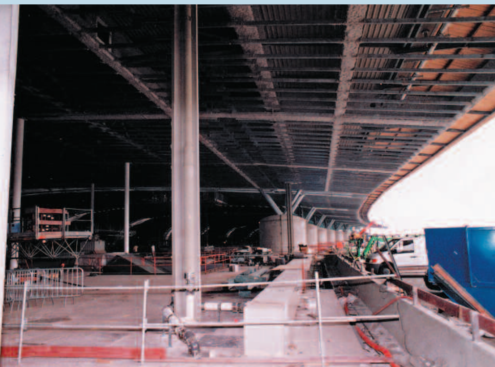
Structure métallique du plafond qui va recevoir les lattes d'ayous. The metallic structure of the ceiling to be finished in obeche ceiling laths. Photo M. Vernay.
