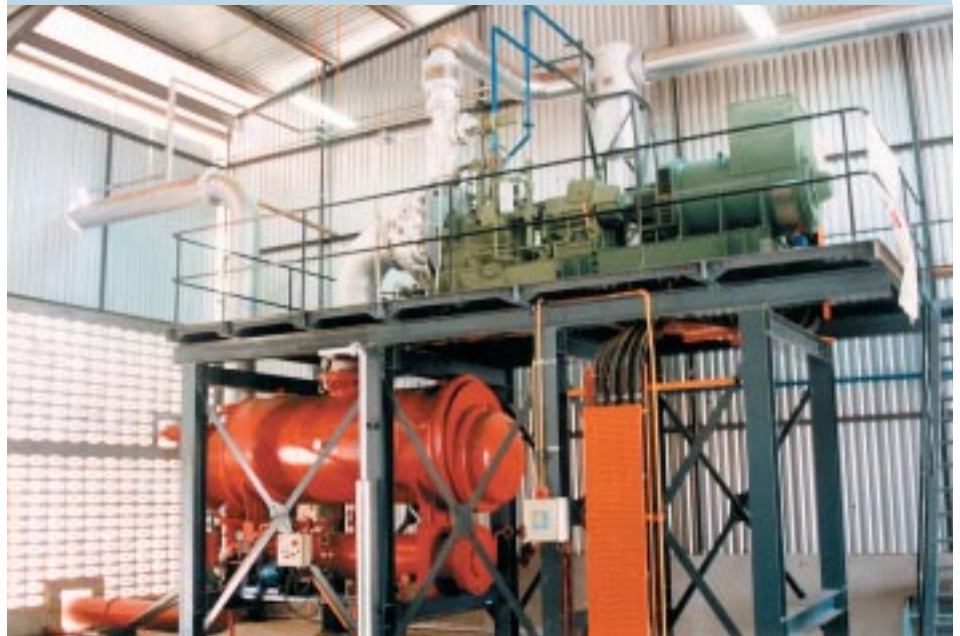
Turbine à condensation Nadrowski (900 kW). Nadrowski condensing turbine (900 kW). Photo P. Girard.
